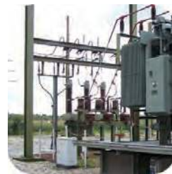
Power Transmission and Distribution
